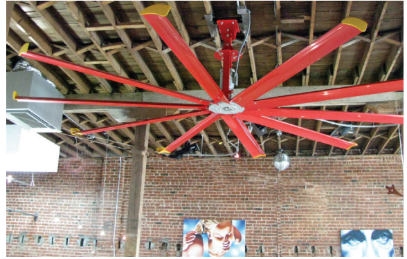
HVLS Fan in warehouse-showroom of Tietsort Design in Oklahoma City.
